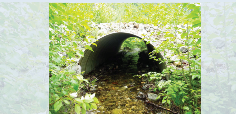
This culvert is the ideal stream simulation scenario. The culvert is larger than the stream width. There is substrate covering at least 25% of the culvert. The culvert has been placed at the same slope of the existing stream bed.
