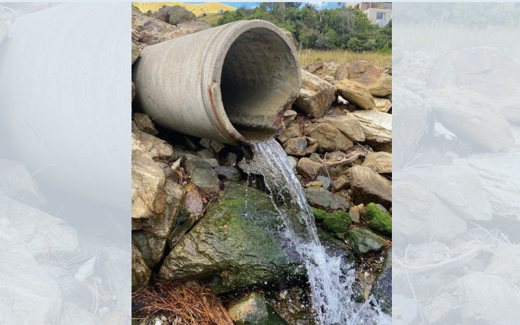
The above culvert has been installed very poorly. The edge is perched, which results in no possible fish passage into the upper catchment.
